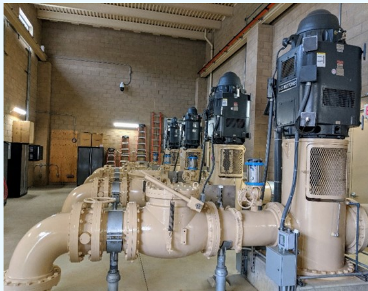
A peek inside the new pump station.
